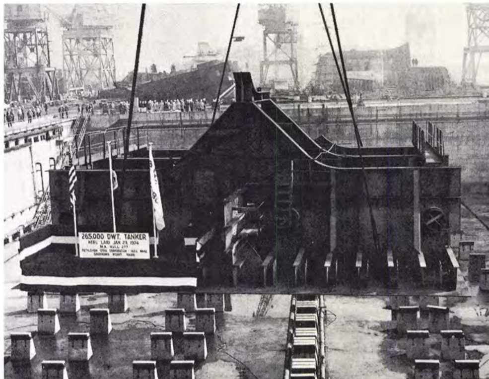
Weighing 187 tons, the first keel section for the largest vessel ever constructed in an American yard—a 265,000-dwt VLCC—is swung into place in the giant building basin of Bethlehem Steel's Sparrows Point shipyard.
