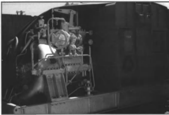
1 Turbogenerator 2000kW Mfg: Westinghouse Model 3S61P537 285psi/417F 3600RPM 10 Stage Generator: Westinghouse 2560kVA 3282Amps 450/3/60
